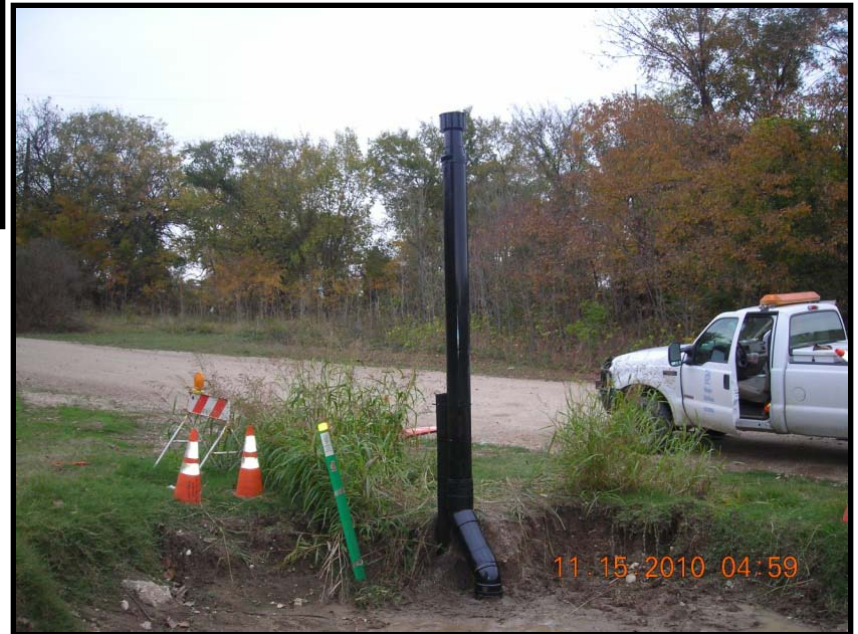
Vent Stack for Wastewater Line
