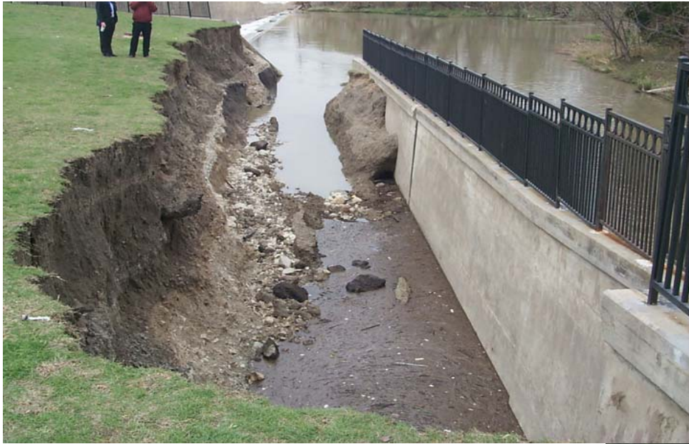
Retaining wall sliding failure on south side of the Spillway
